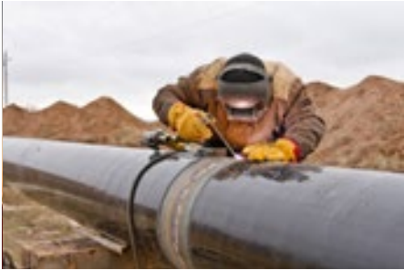
Operation of pipelines
